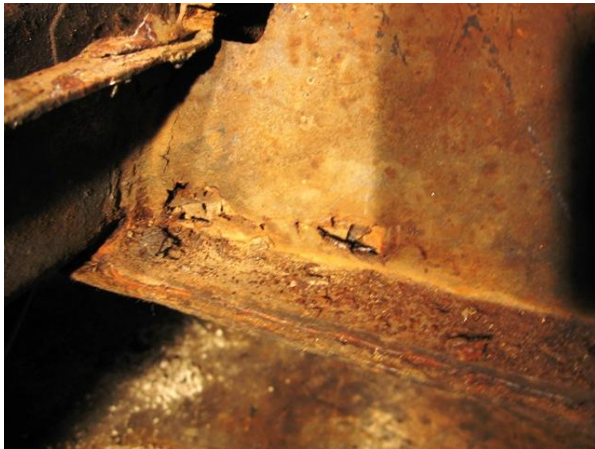
Rust damage at right front torque box
