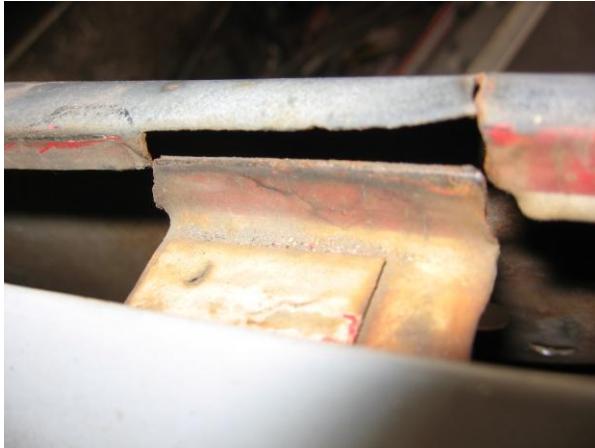
The dreaded fatigue crack! This is on the driver's door.
