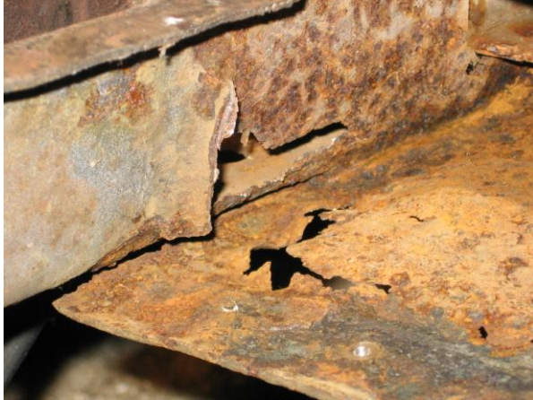
The only frame damage was inside the torque box
