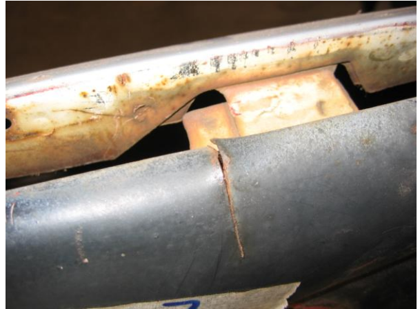
This is the view from the inside of the door. It took a lot of door slamming to create this much damage.
