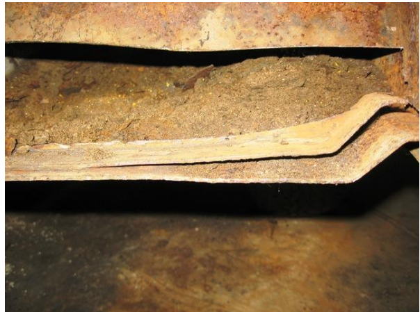
A rusted section of torque box is cut out. Notice the sand that collected inside.
